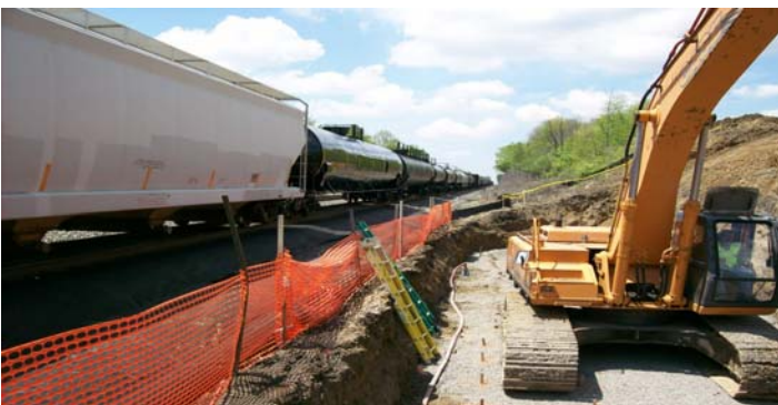
Train at 50 MPH near Quincy foundation.
